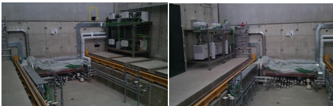
Fig. 2.1.12: SPIDER Cryo-compressors and fore pumping system installed inside the SPIDER Neutron Shield
