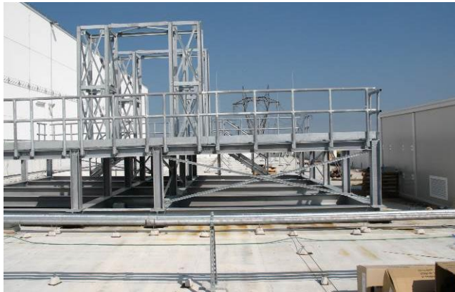
Fig. 2.1.11: The steel structure for support of Cooling Towers on the roof of Building 2
