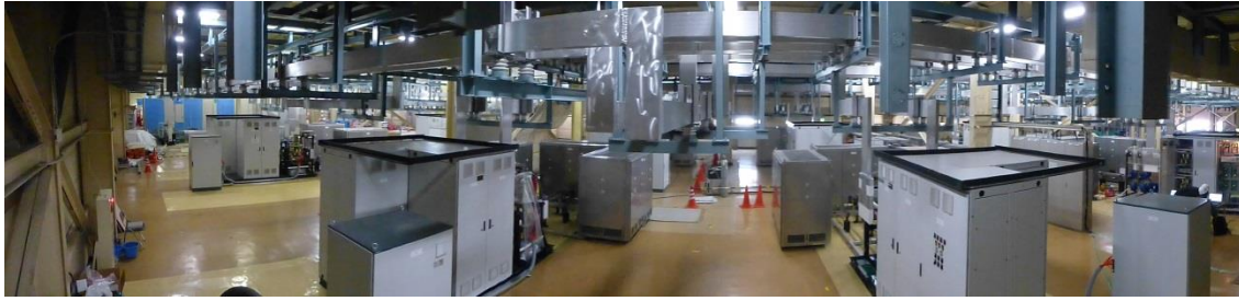
Fig. 4.1.2: View of the QPC units installed in one of the Power Supply Halls at Naka Site
