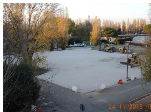
Fig. 2.1.7: Storage area, Area B, used to store components from JADA
