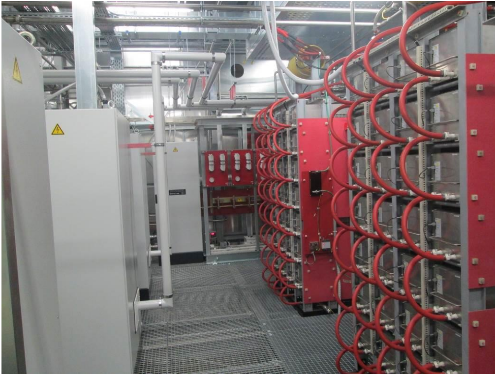
Fig. 2.1.26: ISEPS installation inside the High Voltage Deck
