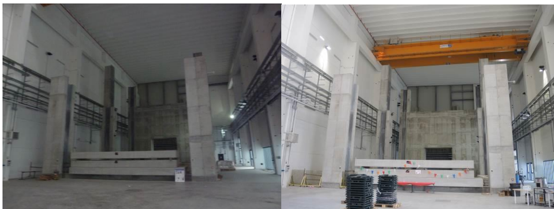
Fig. 2.1.4: PRIMA Site: view of the fixed parts of the MITICA bio-shield inside building
