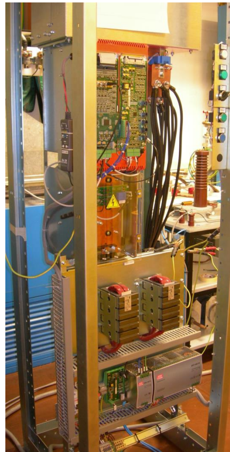
Fig. 4.2.2: RWM-PS inverter prototype installed in the Electric Workshop of the Consorzio
