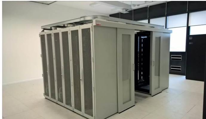
Fig. 2.1.30: SPIDER IT cubicles installed in PRIMA Computer Room
